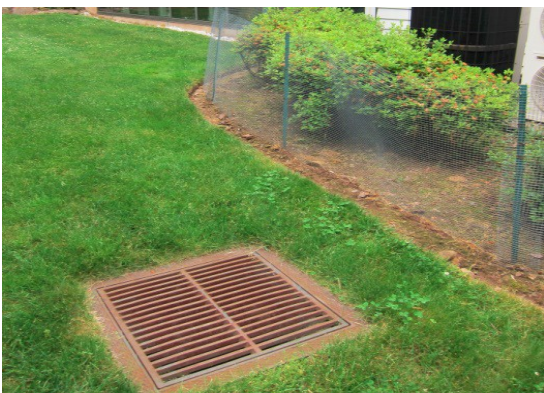
Fig. 2. Dry well installed to receive runoff flowing through a lawn (Source: R. Pitt)
