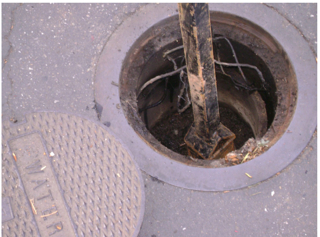
Operating a valve
